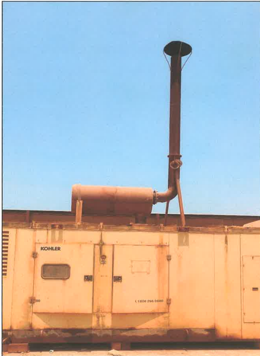
DG Set with Sufficient Stack Height
