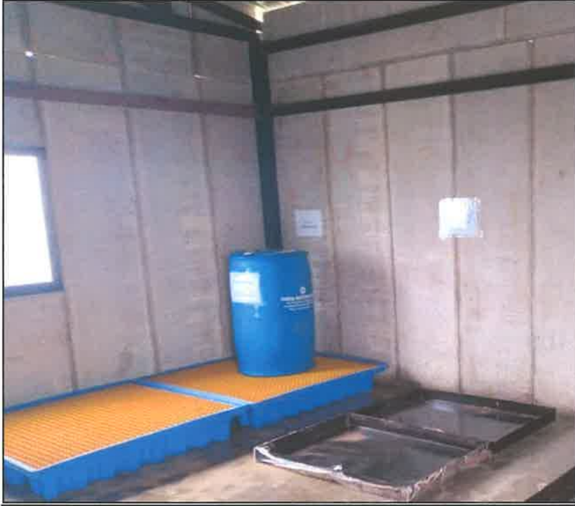
Provision of Secondary Containment at Hazardous Waste Storage Area
